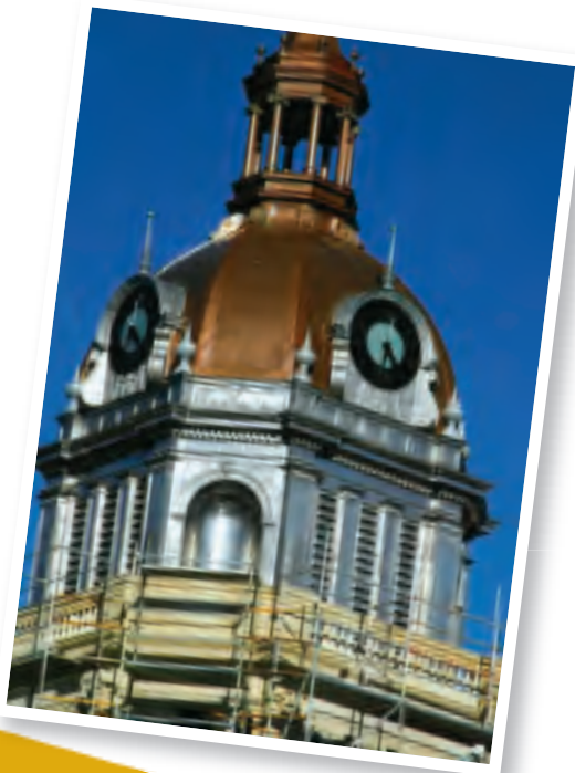
Bourbon County Courthouse Photo courtesy of Steinrock Roofing & Sheet Metal Inc., Louisville, Ky.
